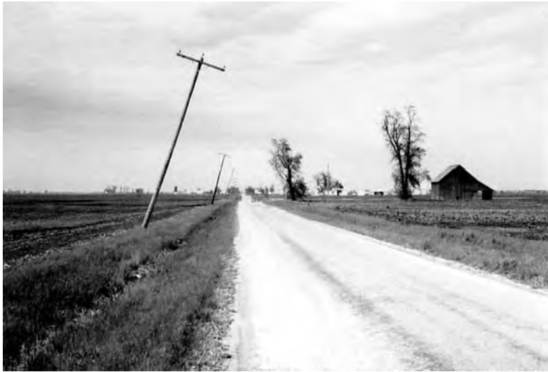
A row of rural power poles partially blown down by a windstorm in Illinois.
