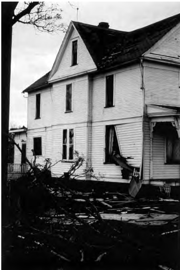
Windblown debris deposited on the side of a house and a fallen tree.
