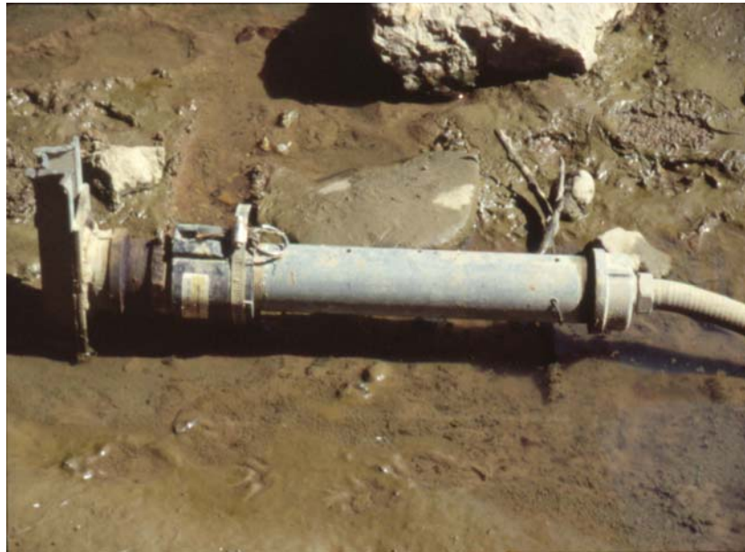
Figure 8. Pressure transducer installed in channel
