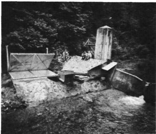
FIG. 5. —SEDIMENT SAMPLER INSTALLED IN FIELD.
