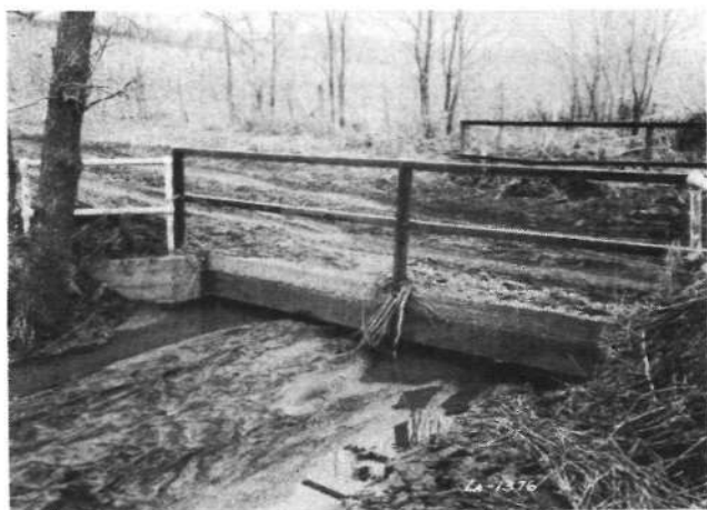
FIG. 13. —CHANNEL BENEATH BRIDGE, CLOGGED WITH SEDIMENT, IOWA.
