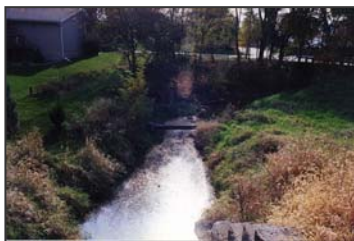
Exposed sewer pipe from stream downcutting
