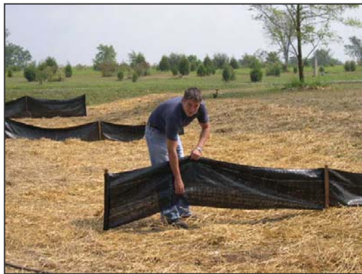
Improperly installed siltation fence in tri-county area
