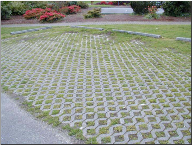
Pervious pavement for stormwater infiltration
