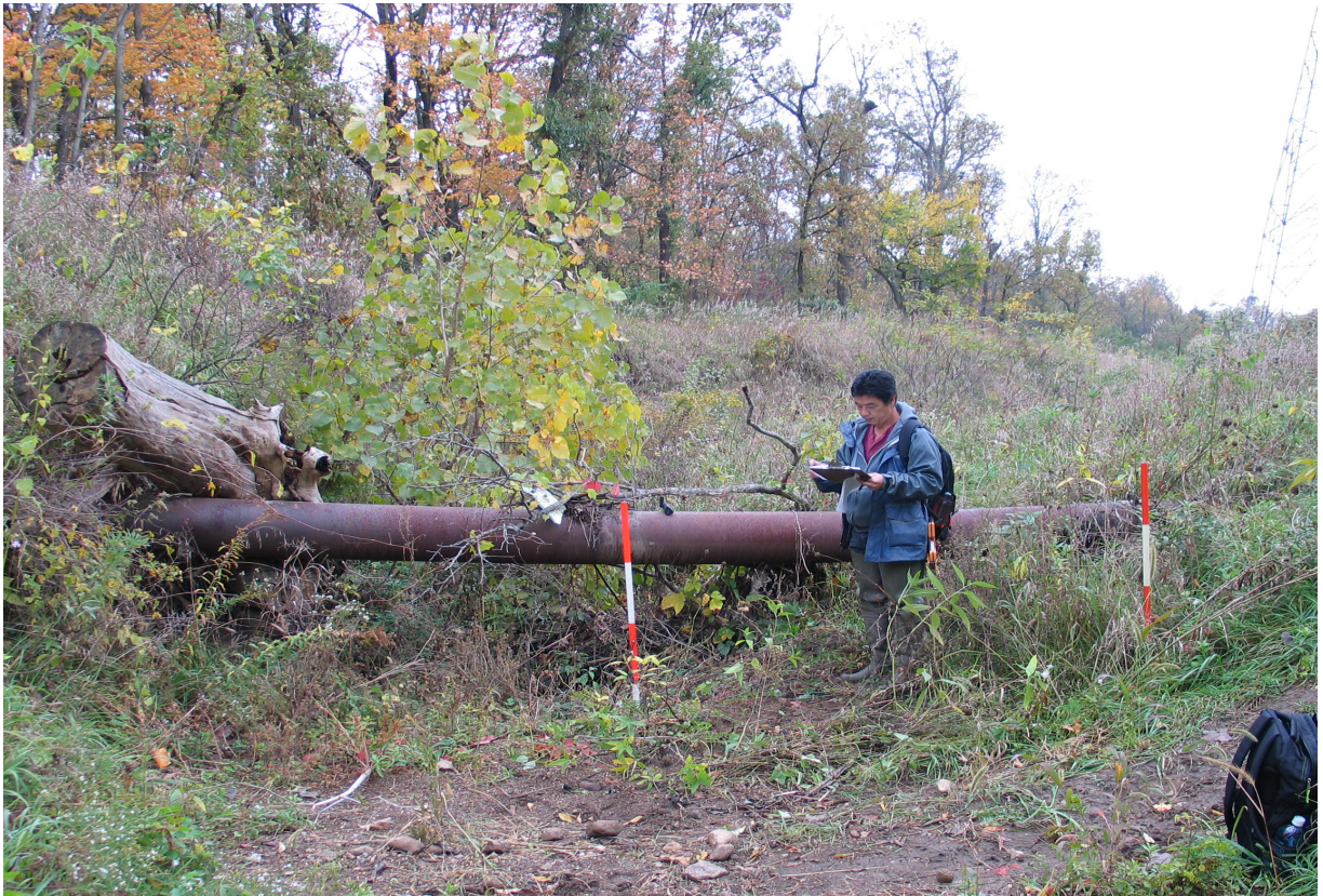
Photo 2. Exposed abandoned gas pipeline along Hallock Creek
