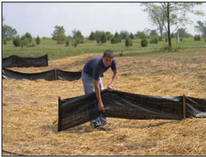
Improperly installed siltation fence in Partridge Creek Watershed
