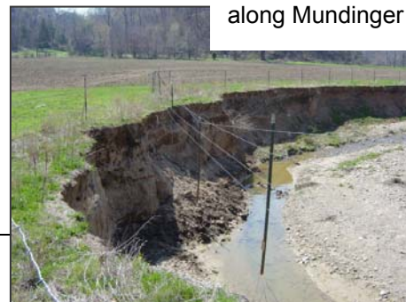
Streambank erosion along Munding Creek
