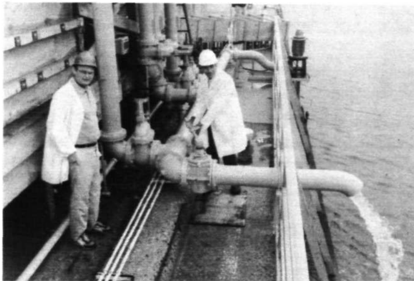
Figure 13. Pumping and piping arrangement, showing flow adjustment via a bypass waste line
